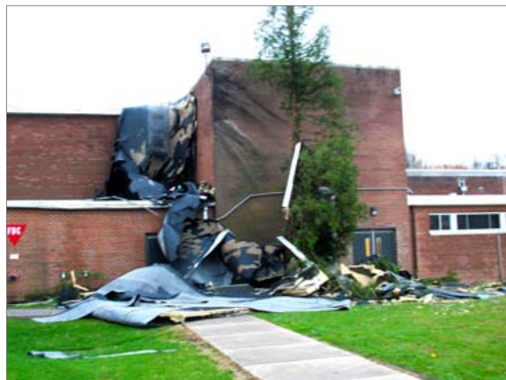
Roofing thrown off of Watchung Hills Regional High school. Photo by: Eric Hatfel
